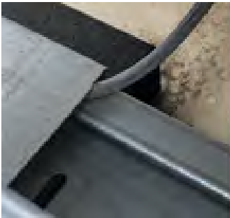
Wires on sharp edges
